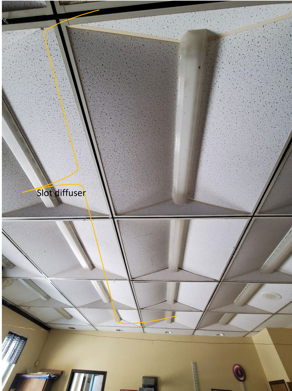
Linear slot diffuser located along the ceiling tiles. This is typical of many classrooms visited.
