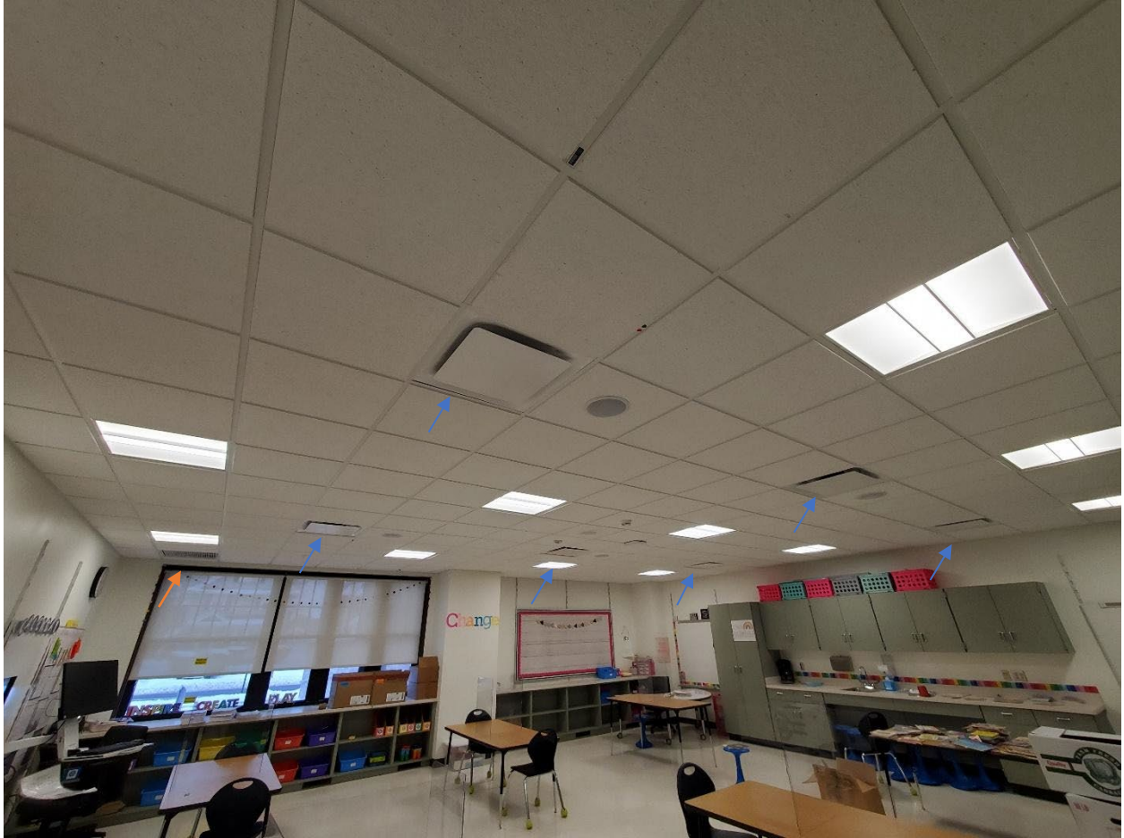
Typical ventilation scheme with 6 supply outlets (blue arrows) and 1 return grille (orange arrow) located on the ceiling
