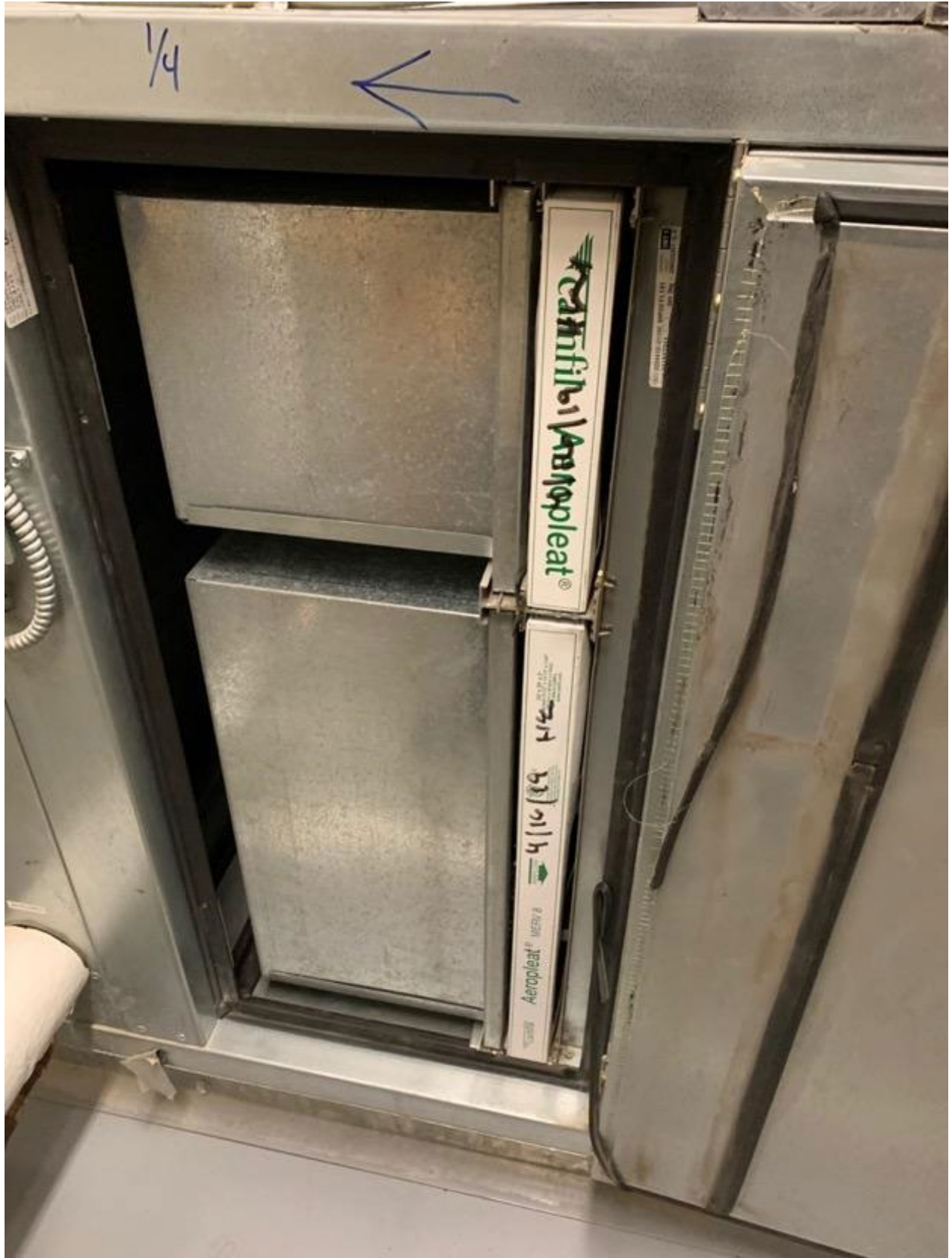
MERV 8 and MERV 15 box filters in the air handlers provide good filtration
