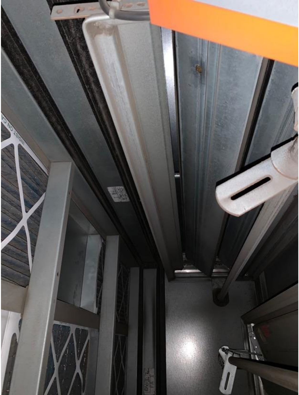
The air handler provides a mix of outside air and return air and filters through MERV 15 filters.
