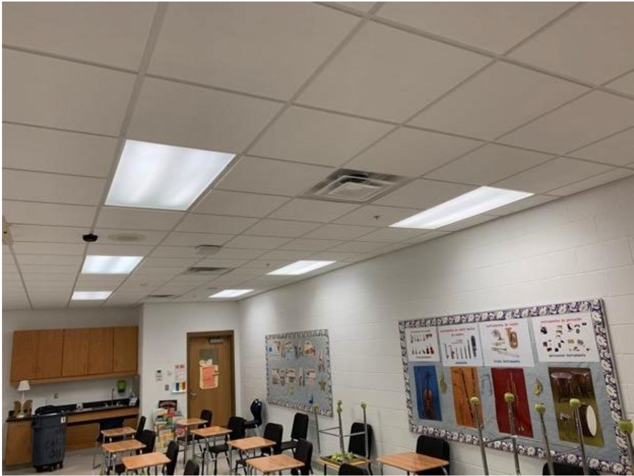
Interior rooms have supply diffusers and are on the central ventilation
