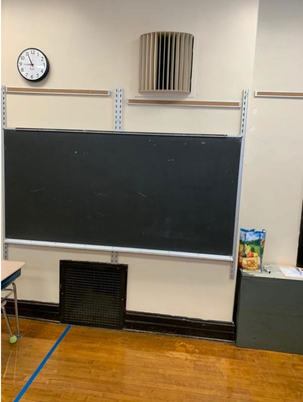
Supply vent in a classroom at ceiling and exhaust at floor
