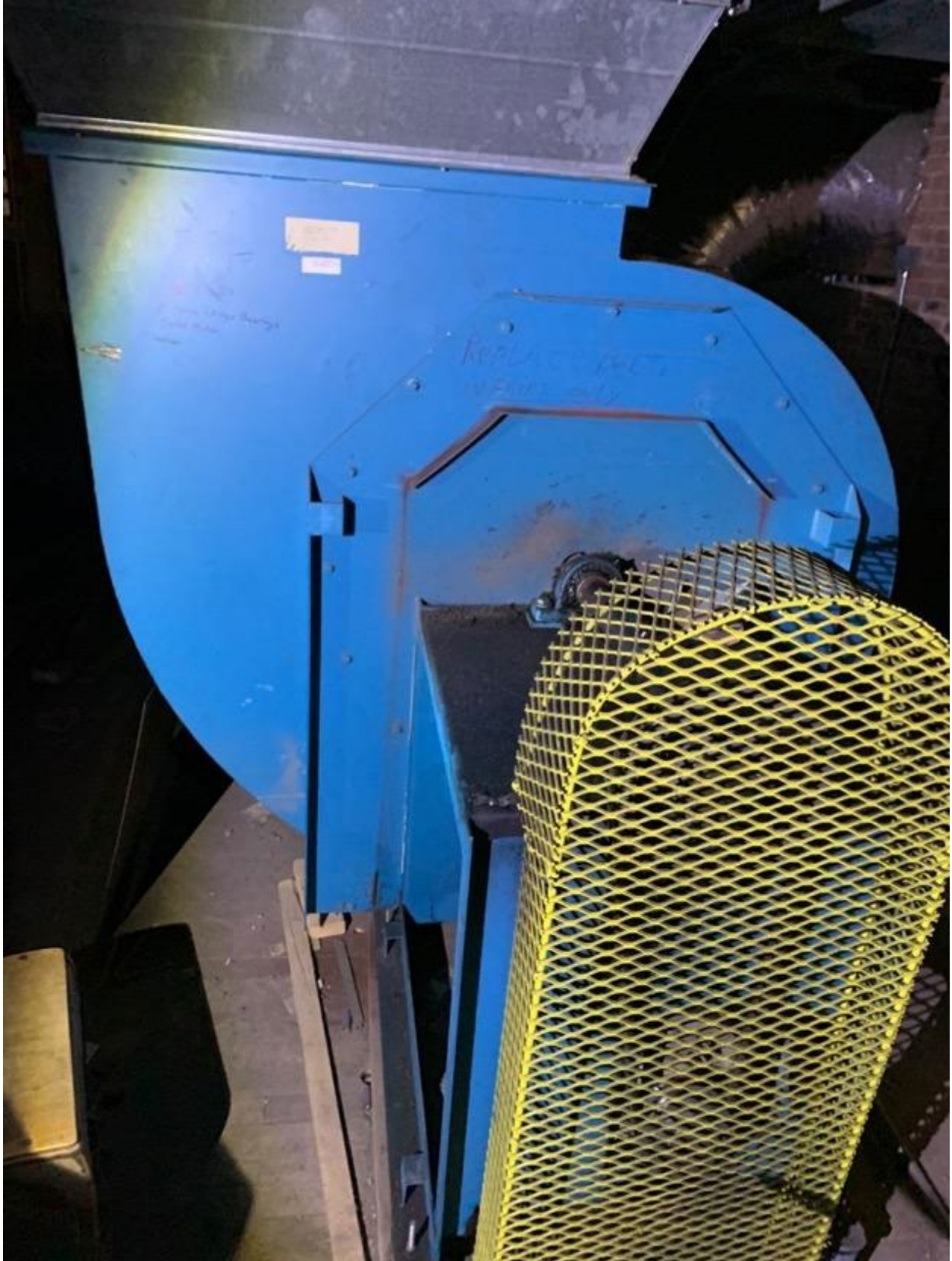
Exhaust fan is running
