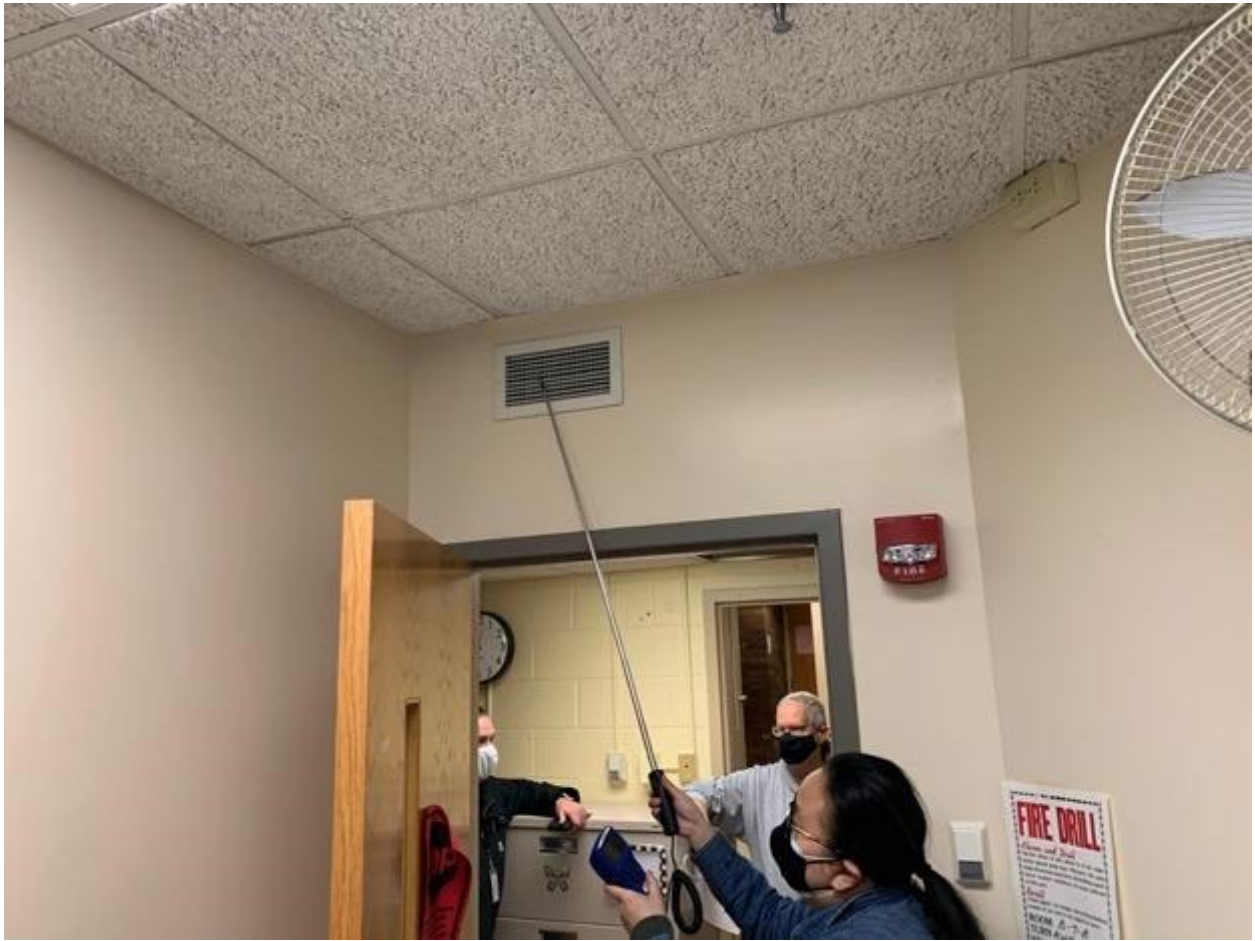
Supply vents provide ventilation air from the blowers
