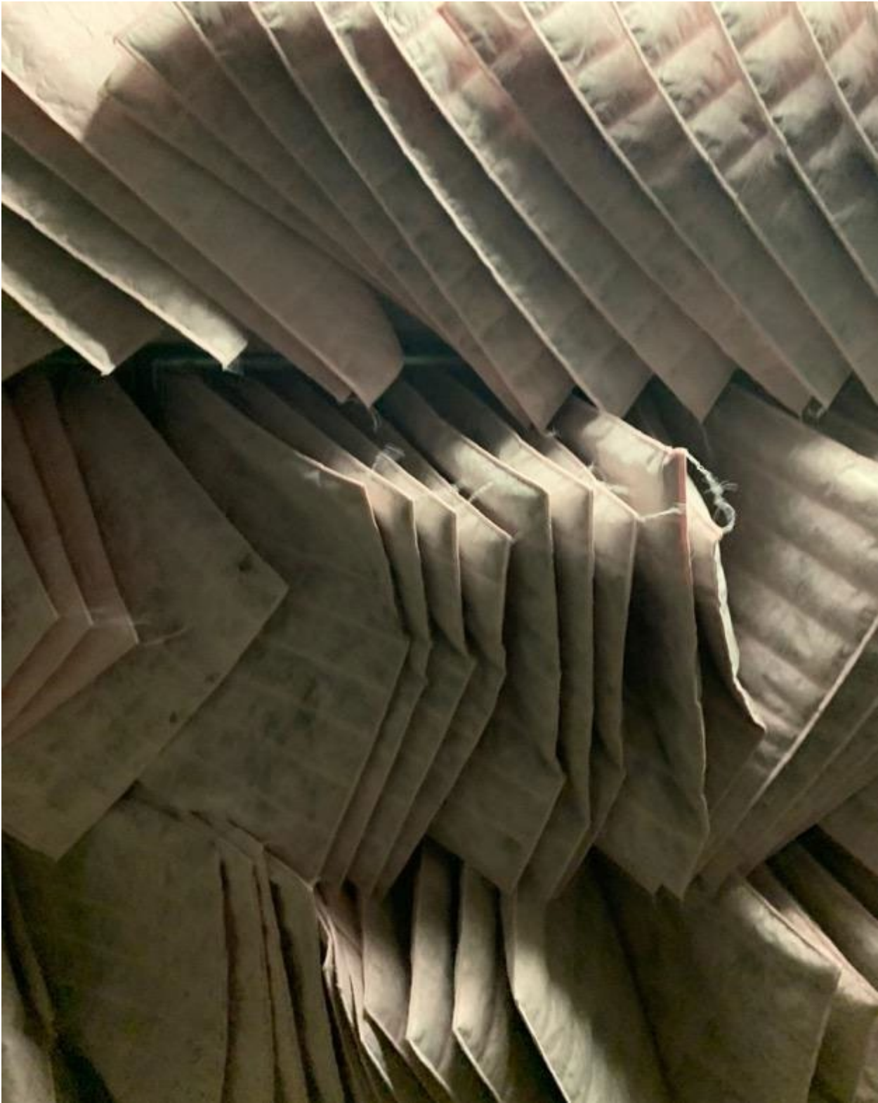
Bag filters on the blower unit
