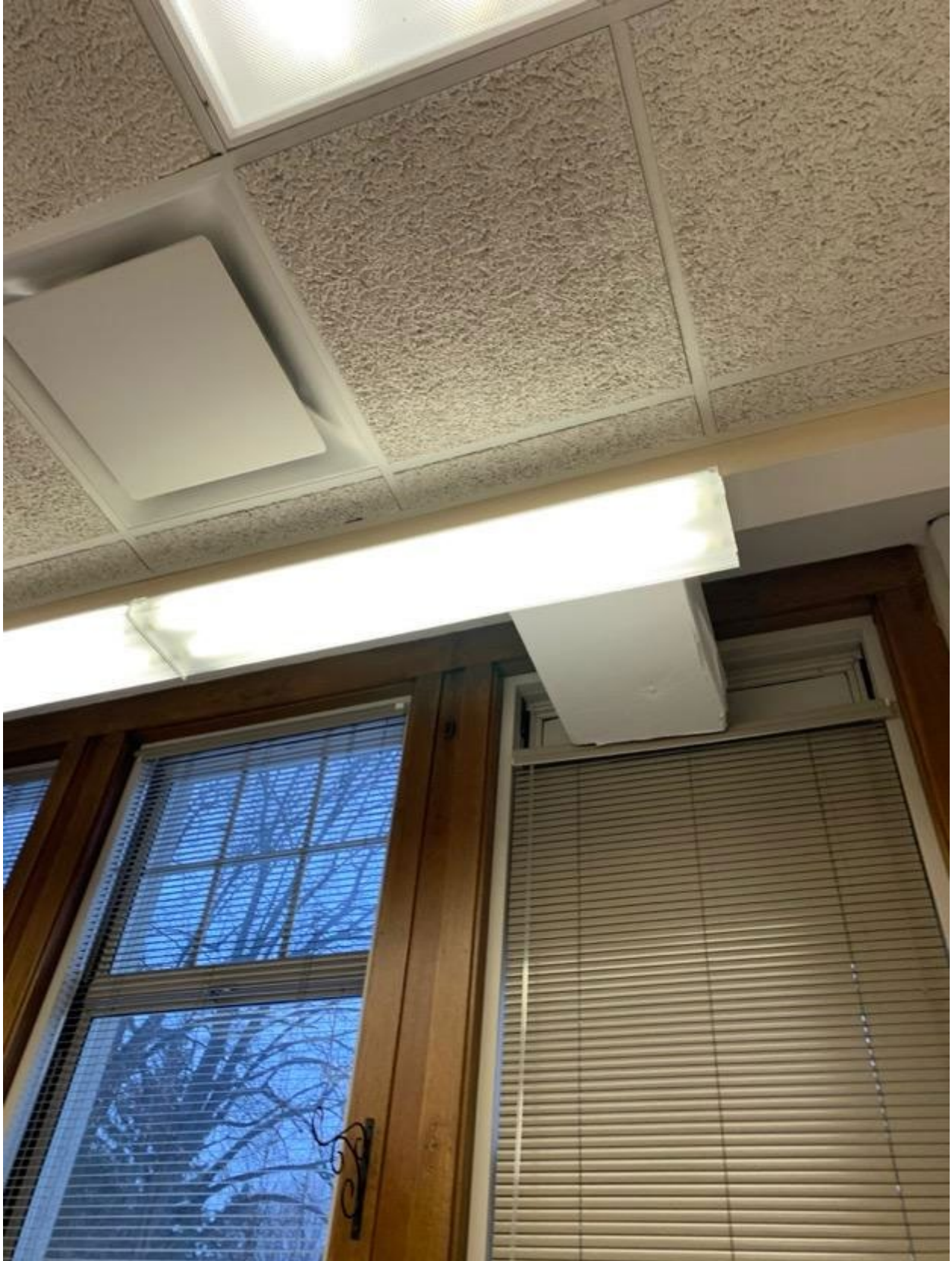
Fresh air duct serving the main office air handler
