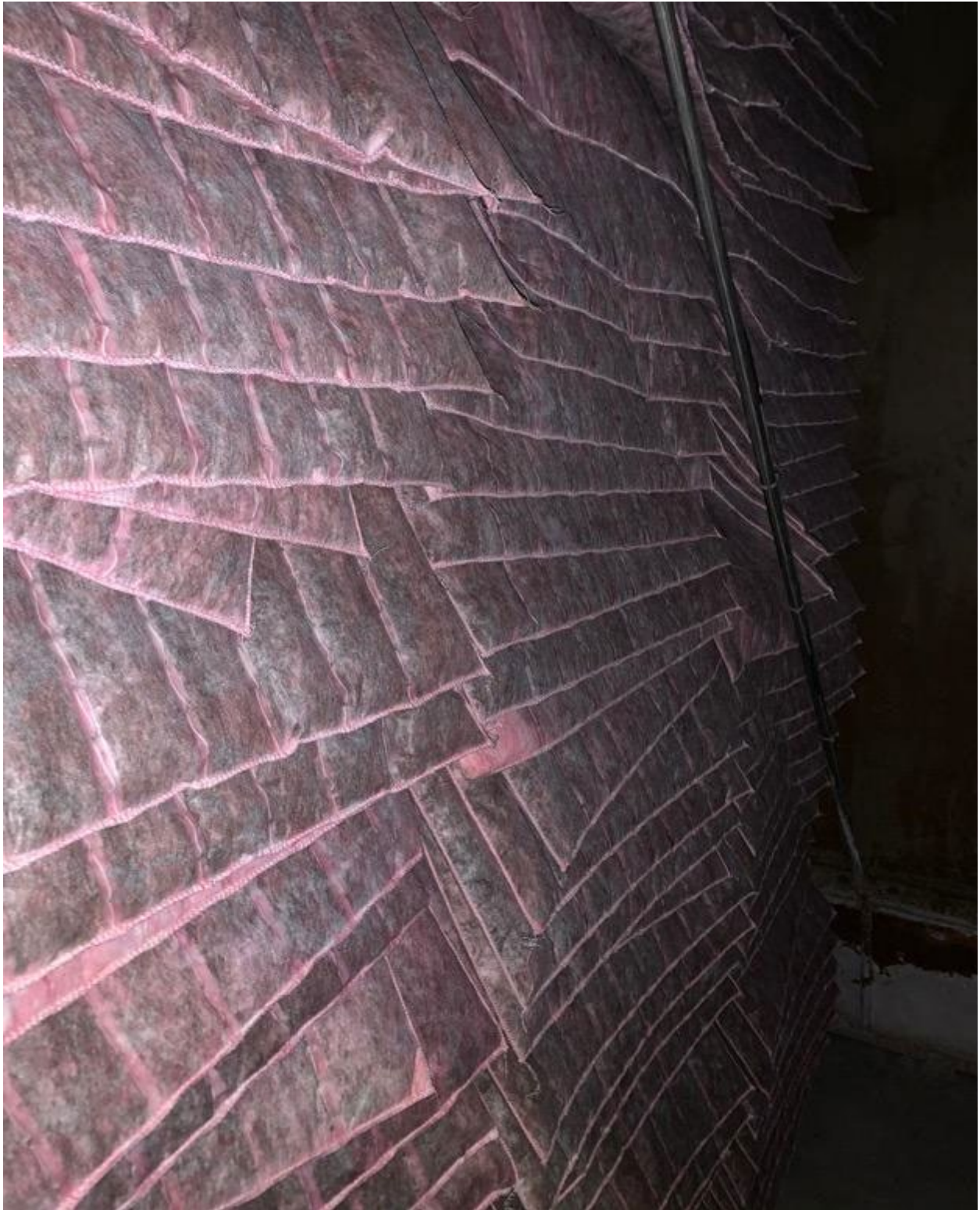
Bag filters on the air handler / blower are efficient
