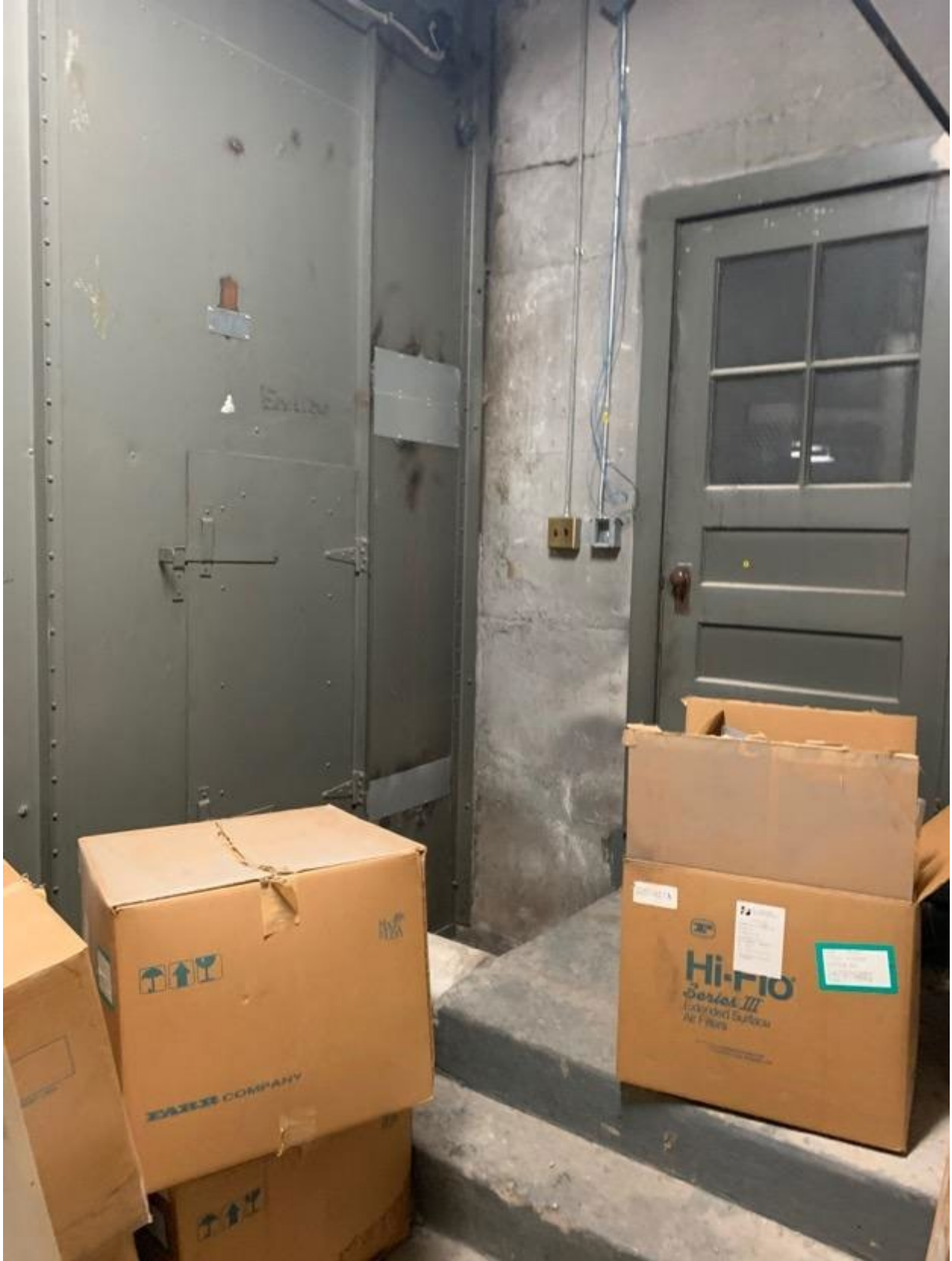
One of the blower units
