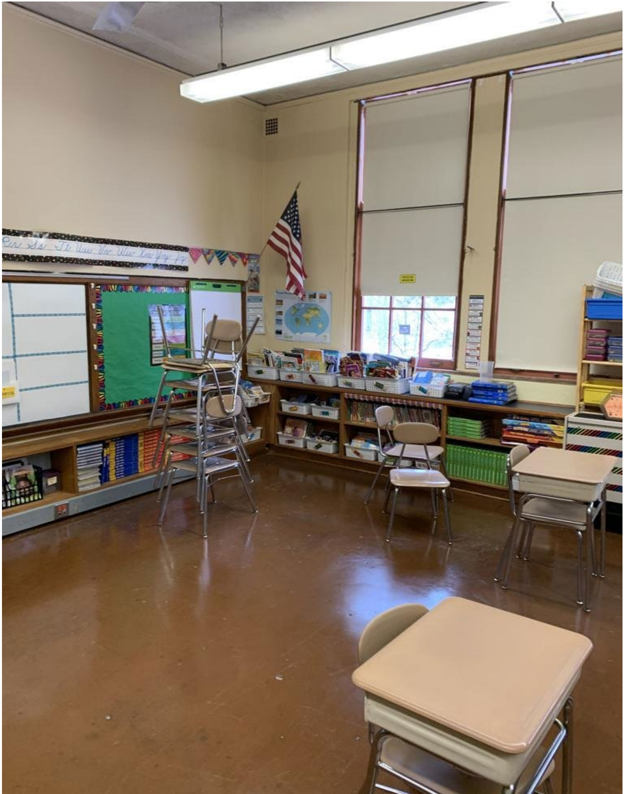
Exhaust vents are also in the upper corners of most rooms
