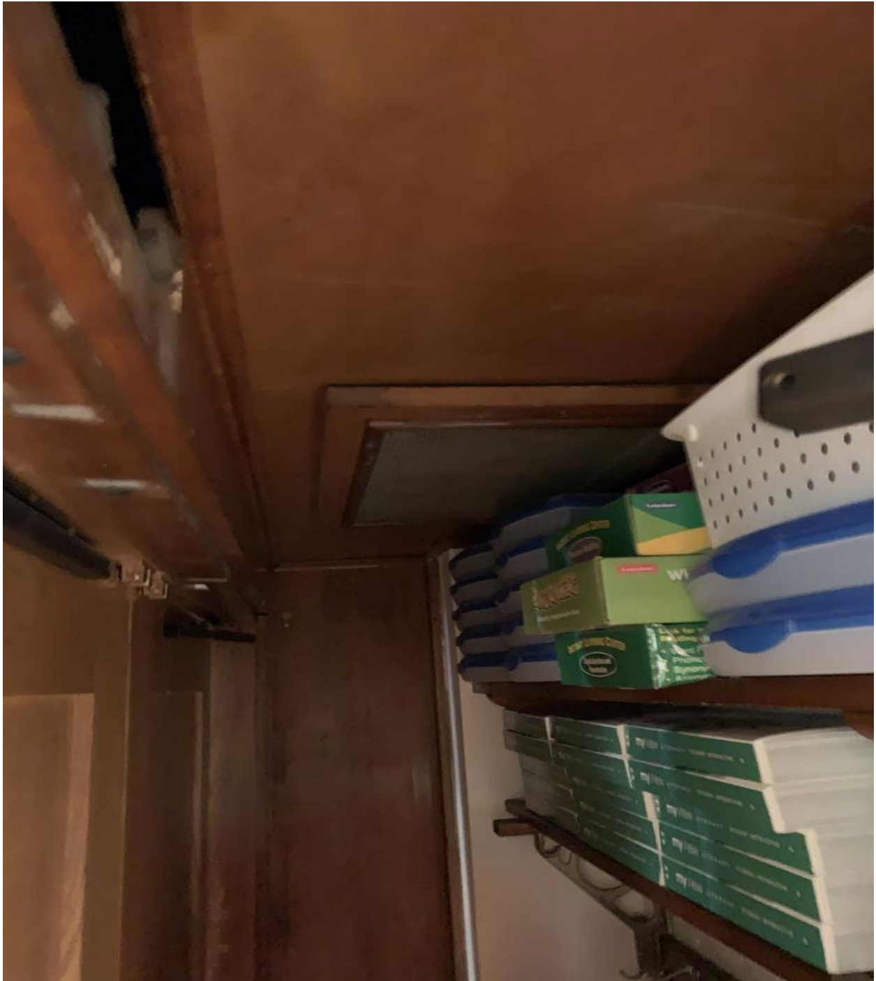
Exhaust in the closets
