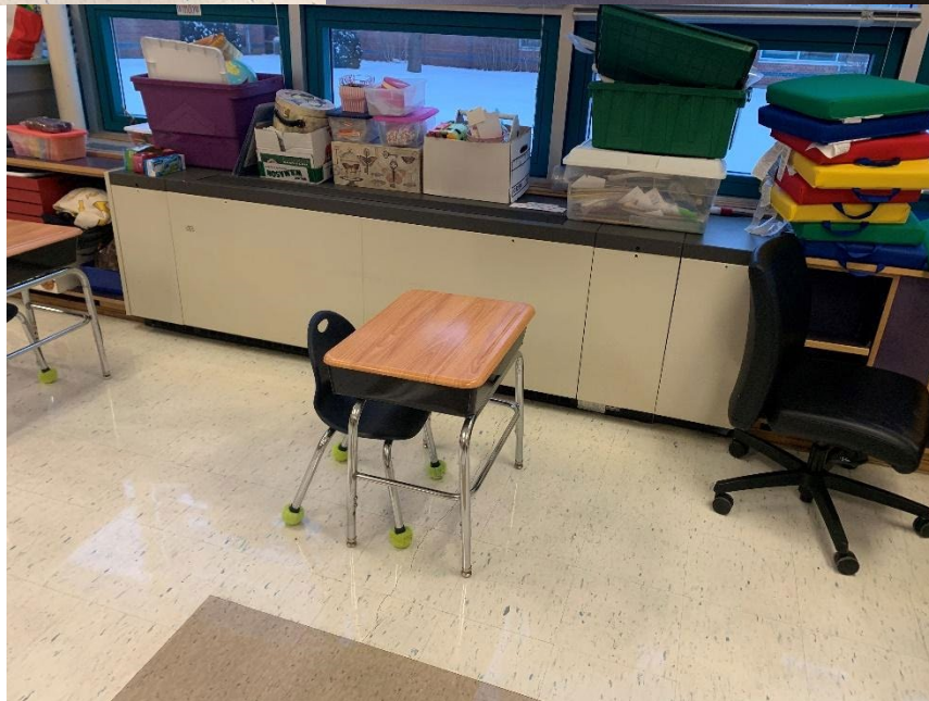
Typical ventilation scheme in a room served by a univent. The univent is located under the windows with a passive return or exhaust in the student closet.
