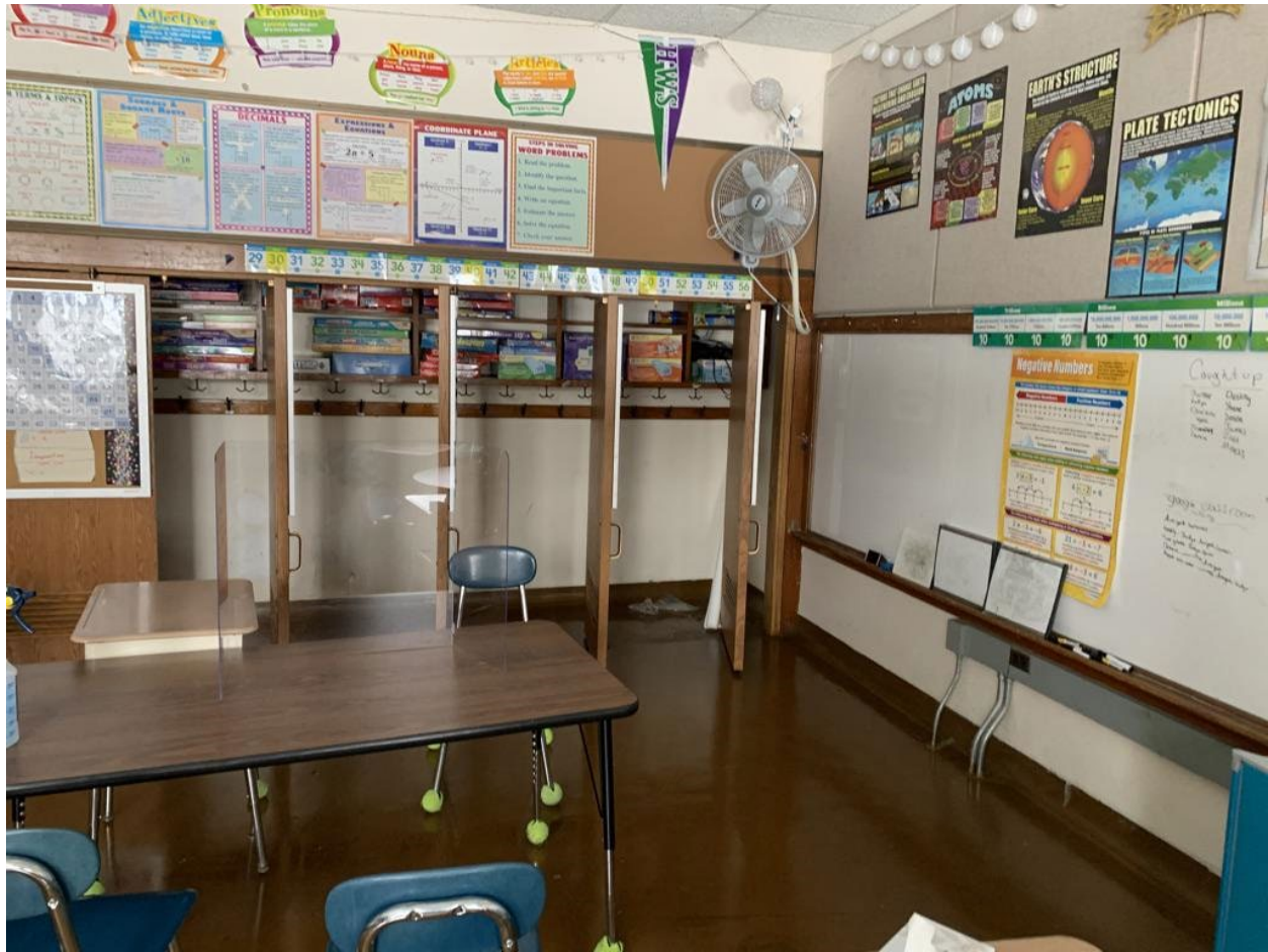
Vents in closet provide natural exhaust ventilation
