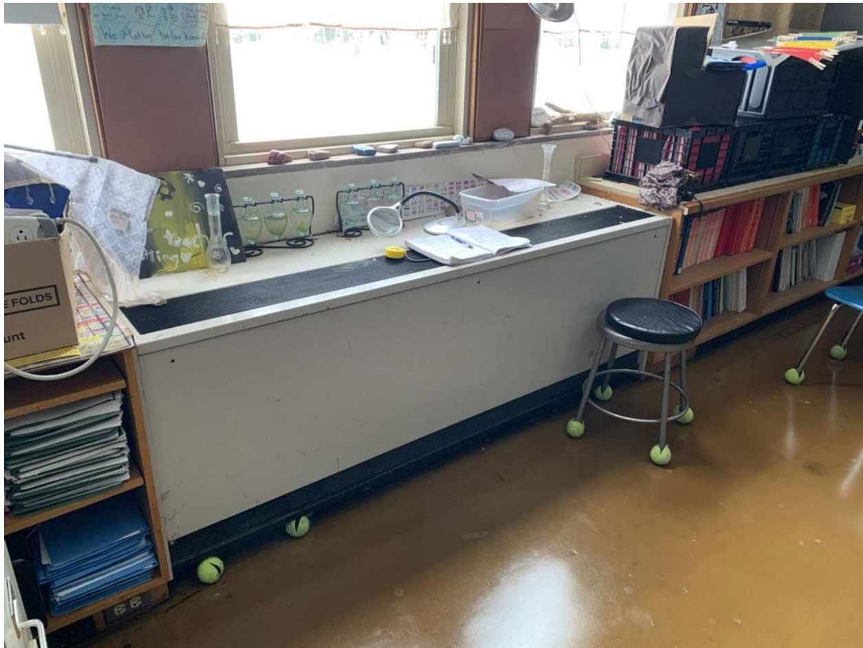
School is heated and ventilated by univents that provide outside air The windows can be opened for natural ventilation
