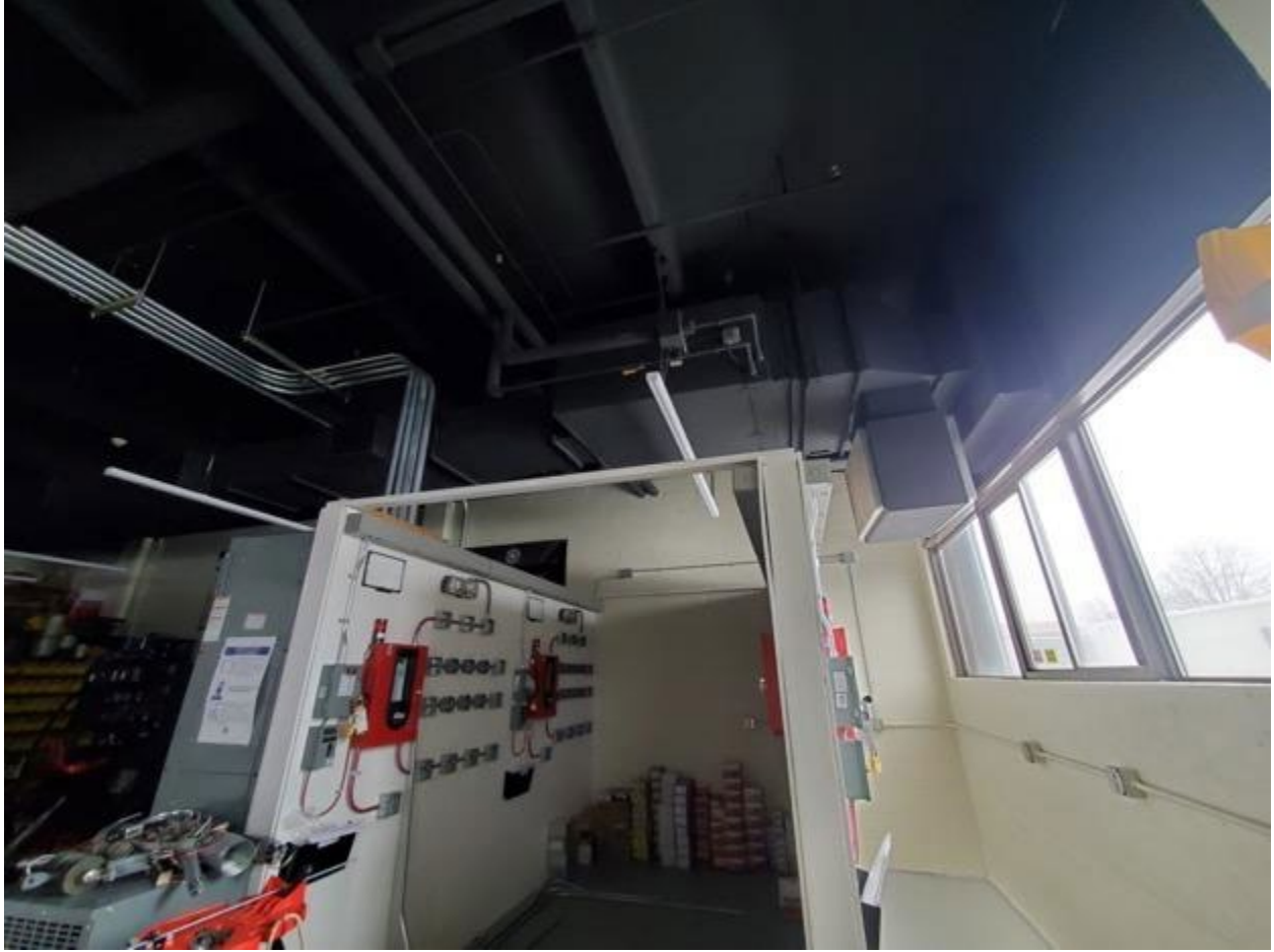
Shop area ventilation unit
