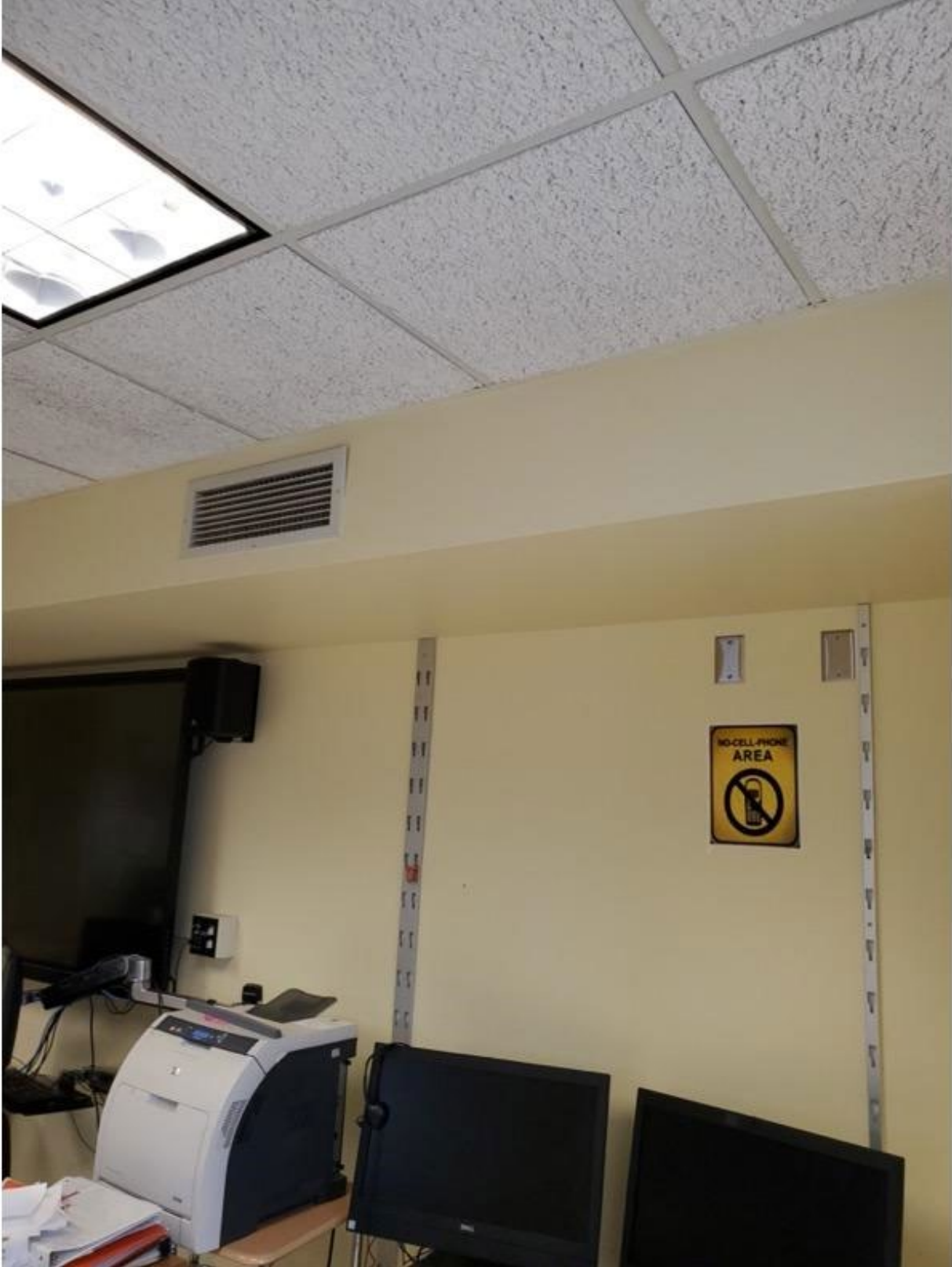
Supply vent from the fan power box
