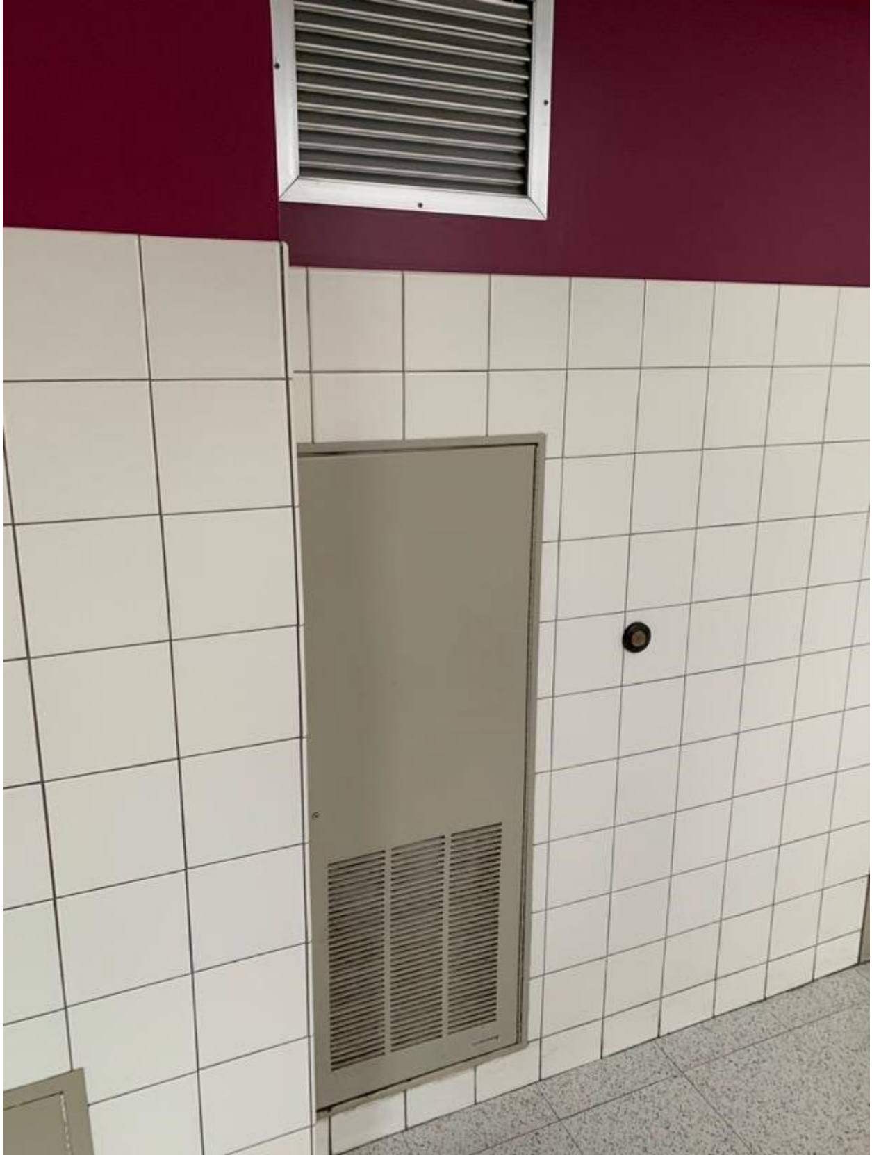
Fan power box in the common hallway
