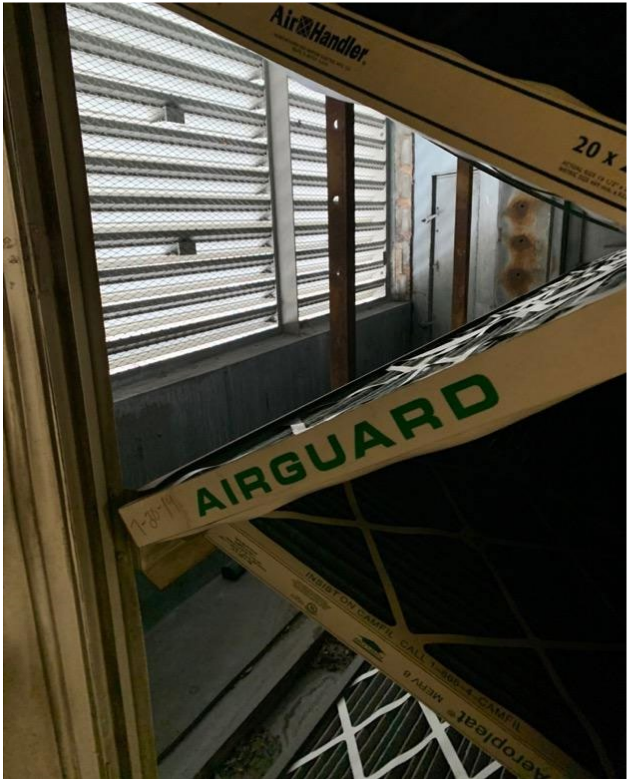
Outside air fan with MERV 8 filters
