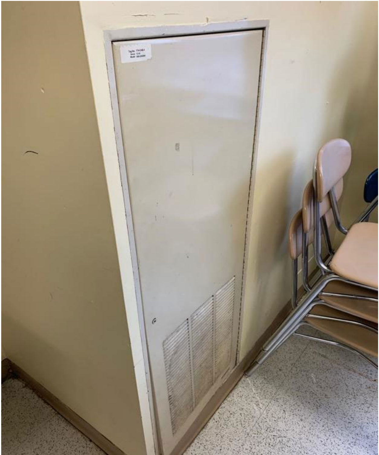
Fan power box in the classroom
