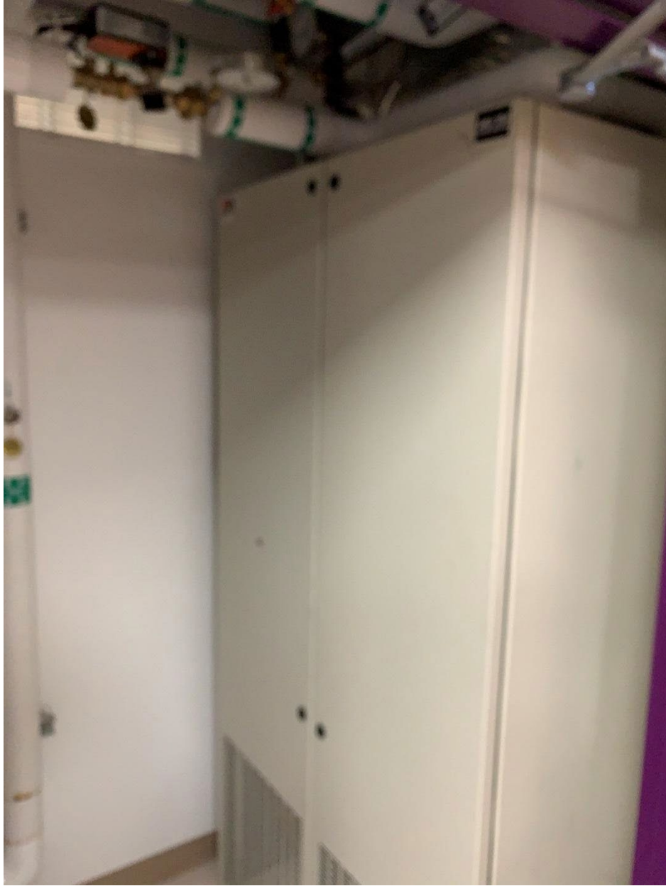
Vertical univent located in Room 254 that serves Room 252 and 254
