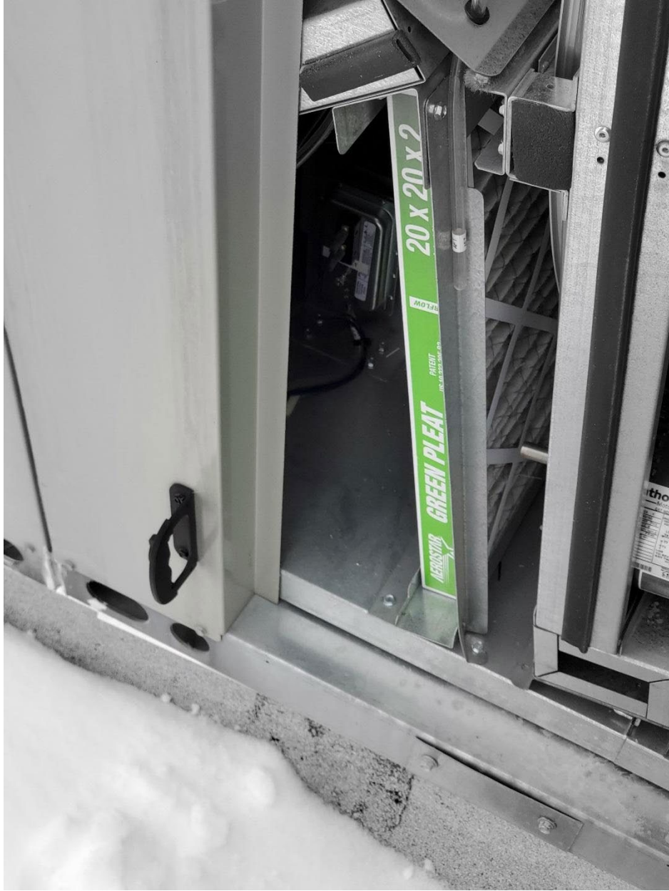
MERV-8 filter inside DOAS, unit is operating to provide maximum outside air
