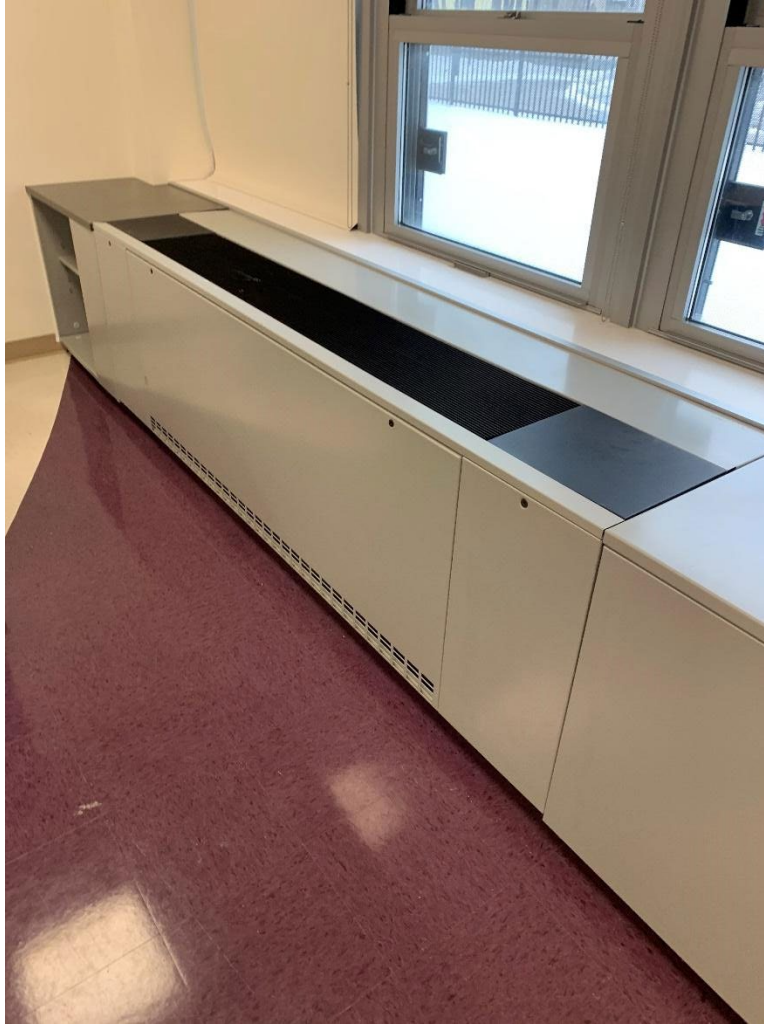
Univent located in Room 101
