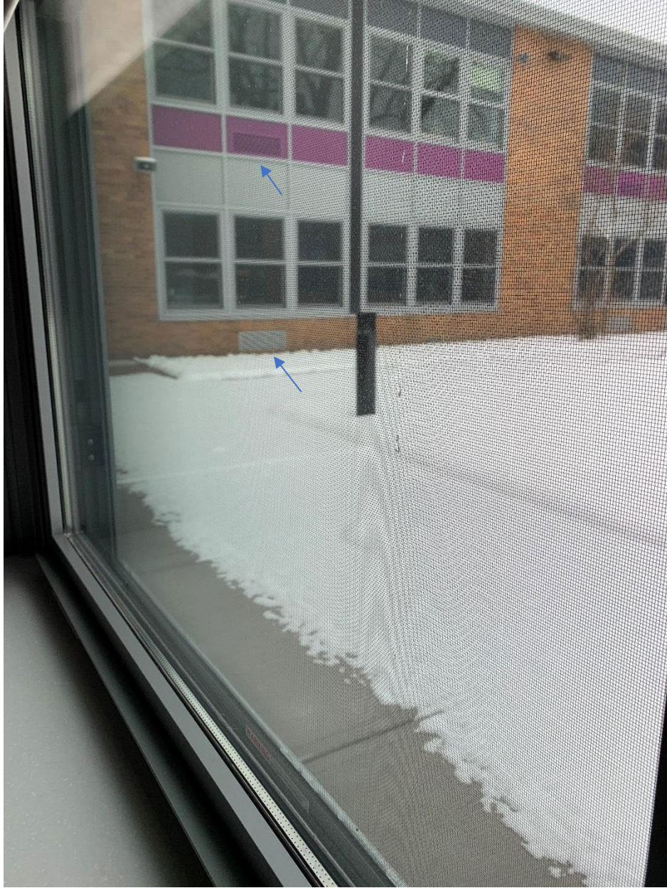
Exterior outside intake grilles seen underneath the windows
